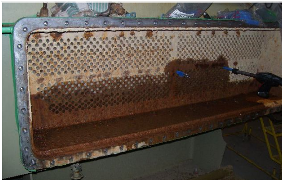
Corroded and damaged heat absorber.
